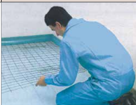
Laying of the support metal mesh, overlapping the sheets by at least 10 cm.
