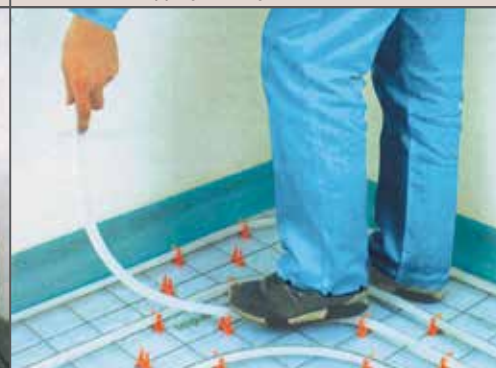
Laying of the pipe on the clips previously fixed to the metal mesh.
