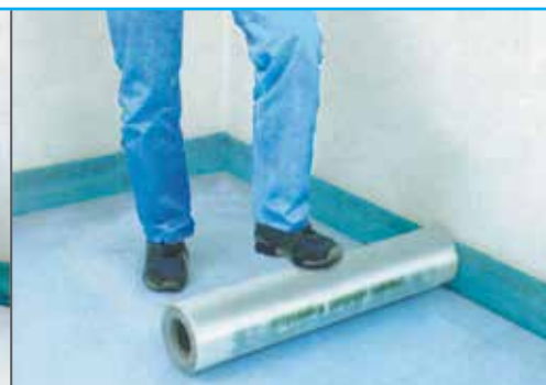
Laying of the protective PE sheet, minimum thickness 0.15 mm, overlapping the edges.
